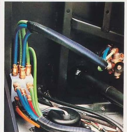
Air junction block
