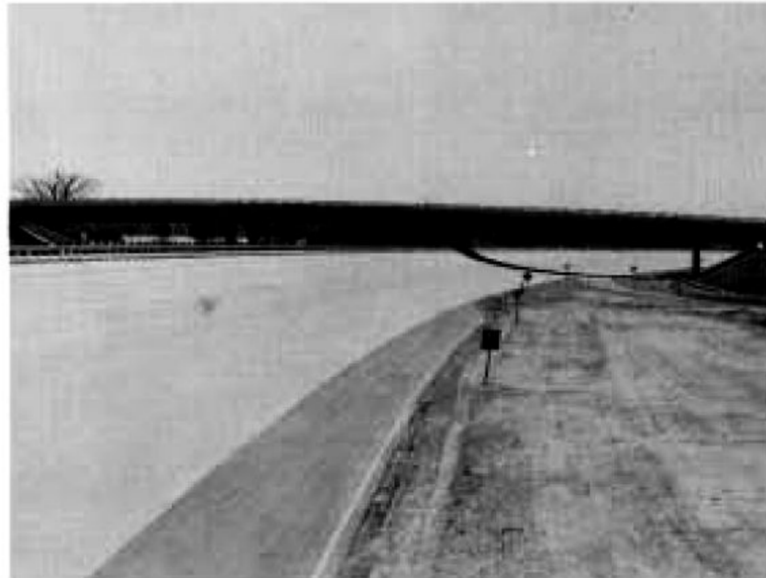
The new 5-mile Circular Test Track is entered from inside the loop via two overpass spans. The one above crosses the new track and the Heavy Vehicle East-West Straightaway. The other span is to the left and overpasses the Oval Test Track and the East-West Straightaway. The front cover is an aerial view of the whole area.
