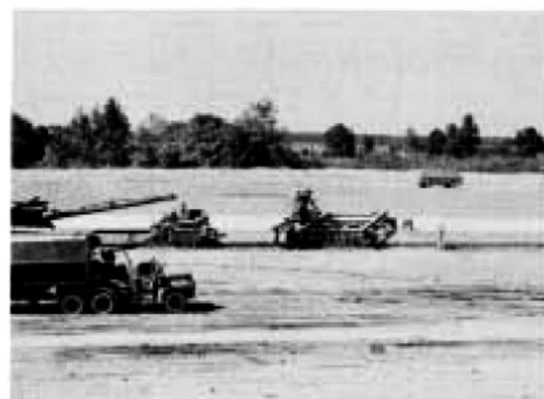
General View of Concrete Laying Operation - 2000 ft per day was normal paving.
