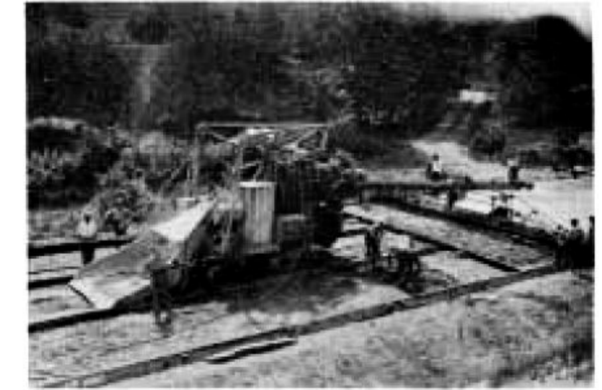
Laying concrete on straight section of Oval Test Track - 300 ft per day was considered very good.
