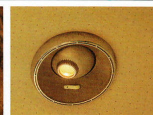
Rear compartment reading lamp.
