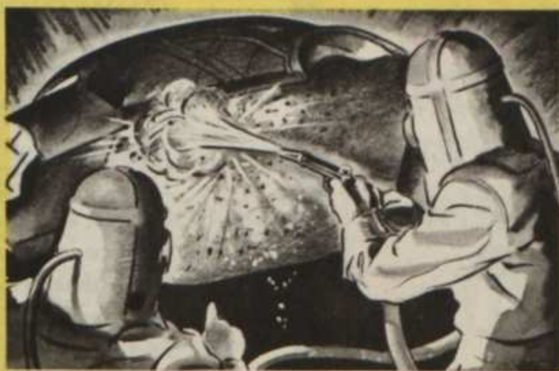
SO NASH-KELVINATOR ENGINEERS perfected a composition containing sand. This is sprayed securely to the floor of the new Nash cars, where they discovered most noise originates—over 50 pounds of it to each car!
